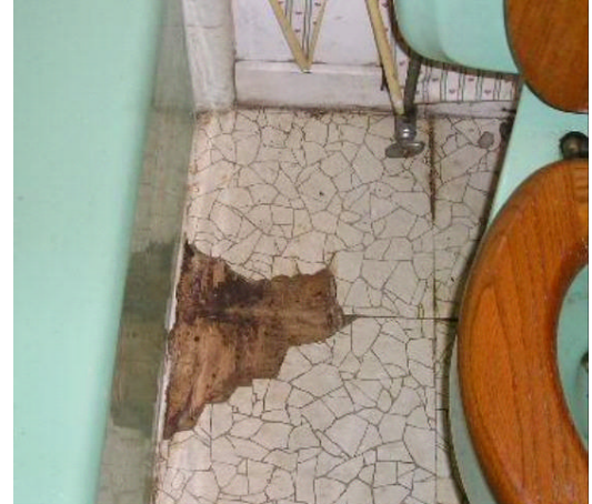
Bathroom floor damage
